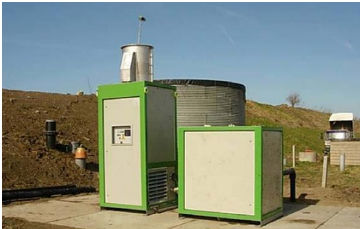
Photos of CEB® 50 unit at landfill
